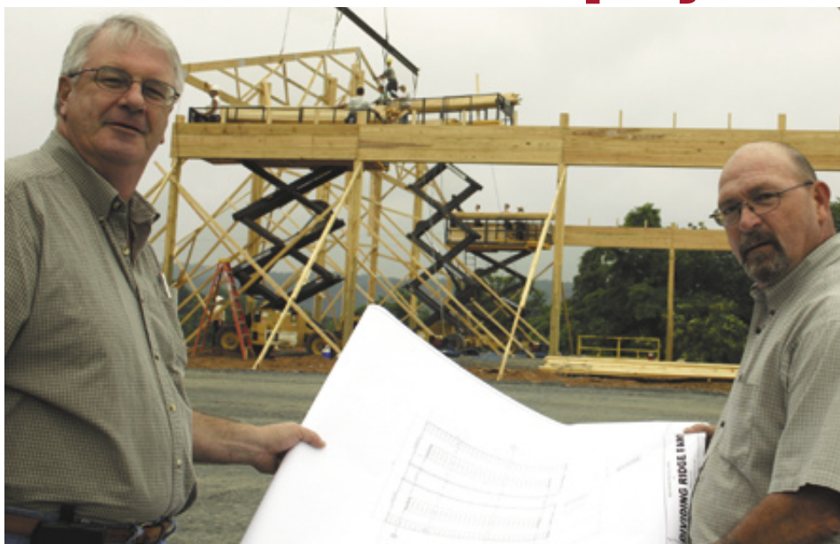
Dean Weidman (left) and Barry Flora show a site plan for a dairy in western Pennsylvania. In the background, trusses are being set on an 80' x 180' hay storage barn at Star Rock Farms Dairy in southeastern Pennsylvania.
